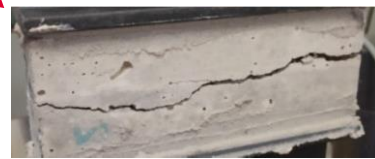
Multiple crack planes
